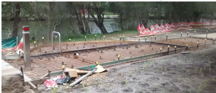
Last section of path on the north of Middle Creek awaits concrete.
